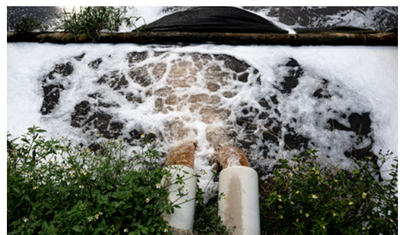
Wastewater discharge area at a textile factory supplying lululemon in Taiwan
