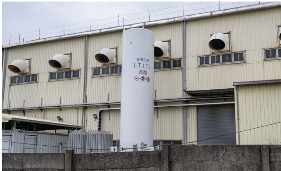
LNG tank outside a textile factory supplying lululemon in Taiwan
